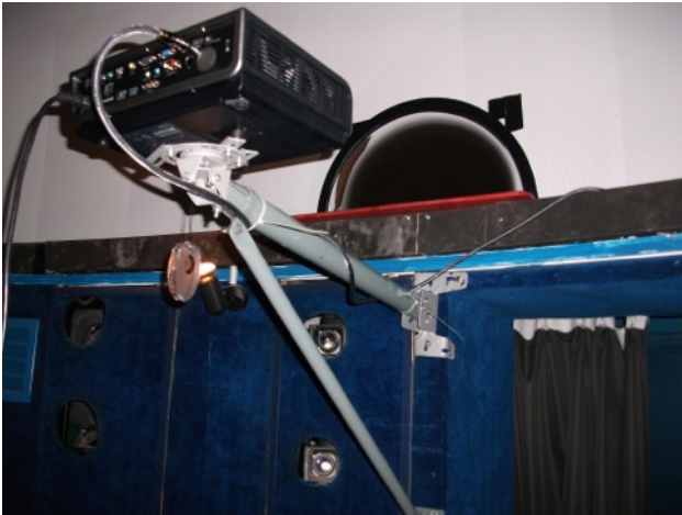
Example of one of many rigs for spherical mirror projection in a fixed dome. Designed on site.
